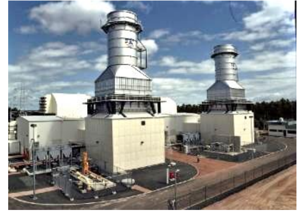
Kemerton Power Station – 300MW
